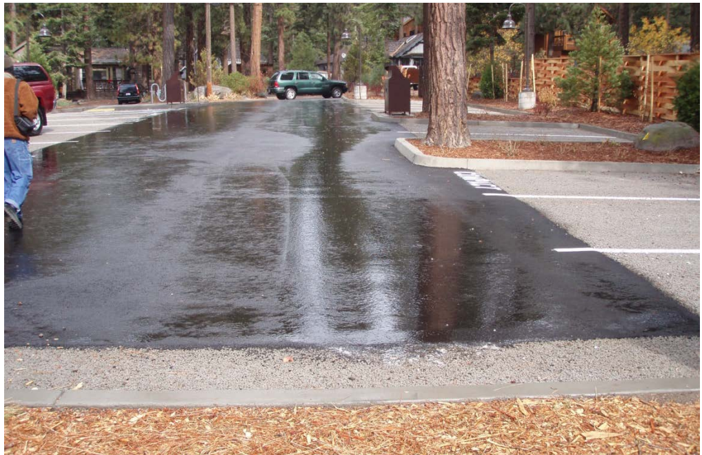
Stormwater runoff from a paved parking lot and the use of pervious pavement along the perimeter and for designated parking stalls.
