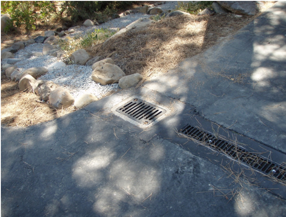
Slotted channel drain with a sediment trap on a residential driveway.
