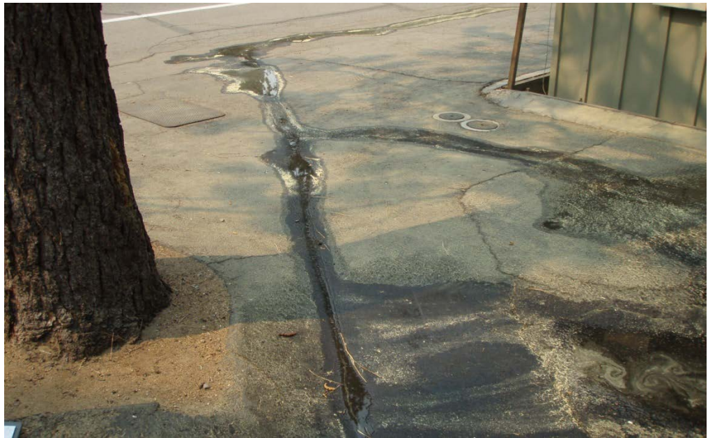
Running a hose on a property can help identify flow patterns and discharge locations.
