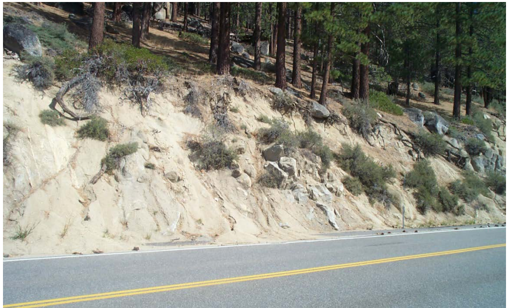
This cut slope is eroding, delivering sediment to the paved roadway.
