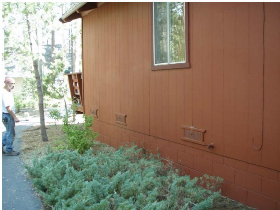
Although drought tolerant and able to withstand the Lake Tahoe Region's winters, junipers are highly flammable woody vegetation and can burn intensely if ignited. Junipers should not be planted next to structures.
