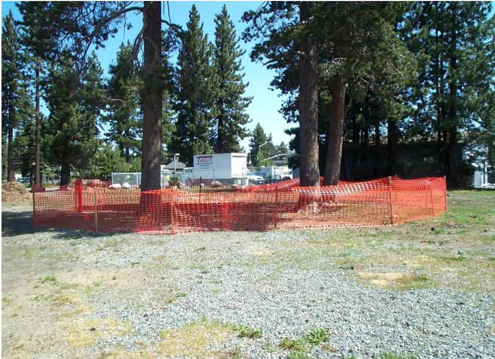
Extend protective fencing to the width of the dripline to ensure adequate protection of roots.
