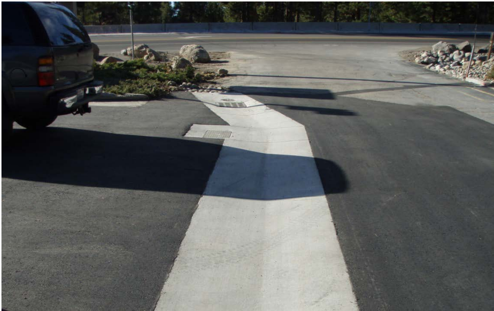
Concrete swale on a commercial site conveys stormwater to a drain inlet.
