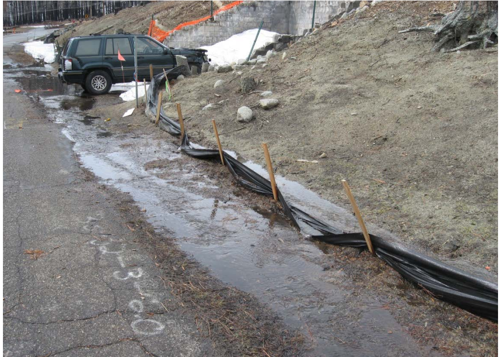
This silt fence is not functioning and needs maintenance.
