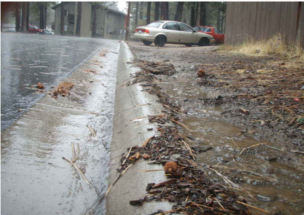
This rolled curb is conveying stormwater runoff from the parking lot but it not preventing vehicle encroachment to the unpaved shoulder.
